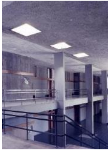
Figure 26 Two main ceiling types at the Faculty of Architecture building selected for modelling.
